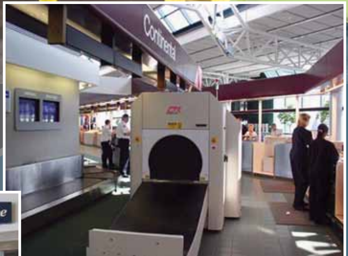
In-line explosive detection system, before
